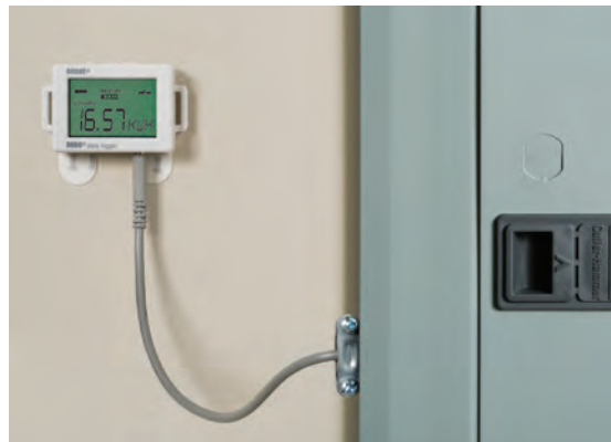
HOB0 UX90-001 State data logger monitoring plug load at the panel
